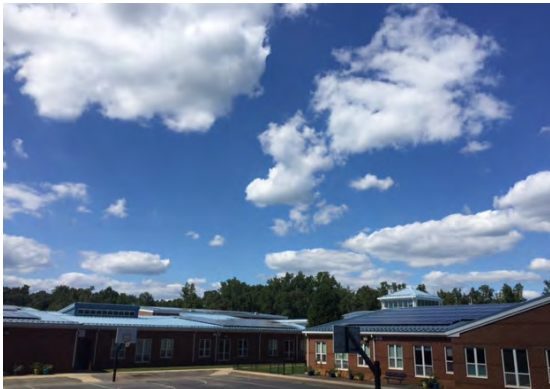
Rooftop solar installation at Baker-Butler Elementary School in Albemarle County.
