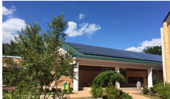
Rooftop solar installation at Mary Carr Greer Elementary School in Albemarle County.
