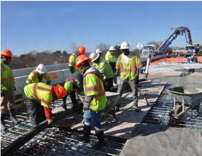
Crews pour concrete for the new deck of the U.S. 17 Southbound bridge over Norfolk Southern Railroad and Route 805.
