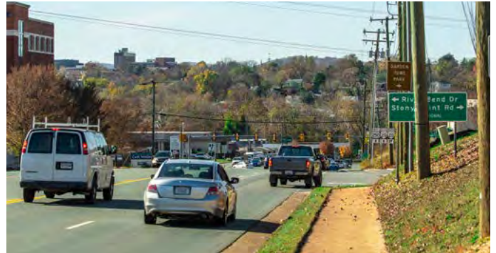
Two SMART SCALE projects are being bundled to reconstruct a segment of U.S. 250 (Richmond Road) between Route 20 (Stony Point Road) and Rolkin Road at Pantops.
