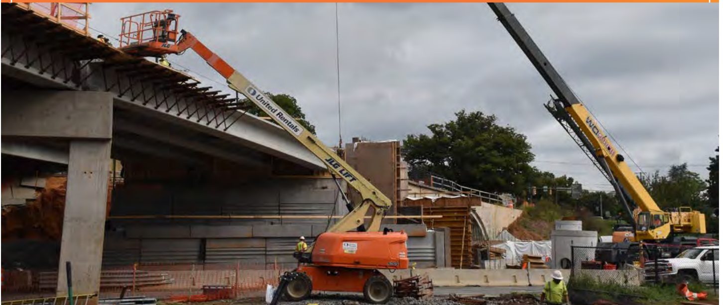
The aging Belmont Bridge in Charlottesville is being replaced through a $35.4 million project. Construction is under way; completion is scheduled by January 2024.
